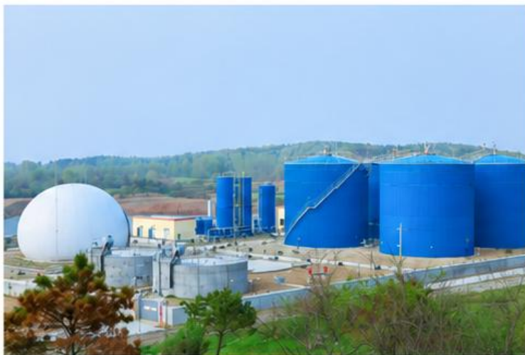
COFCO Wuhan Guangshui pig manure project
