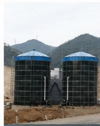
Landfill leachate UASB reactor
